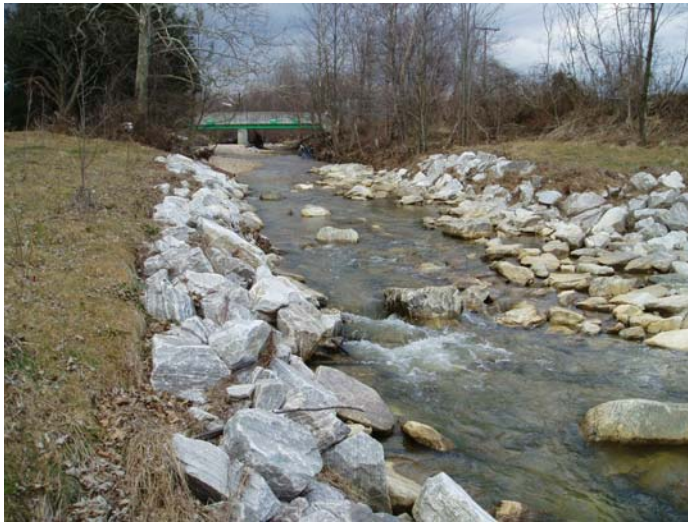
Recently Completed Little Paint Branch Fish Passage Project at the Beltsville Agricultural Research Center
